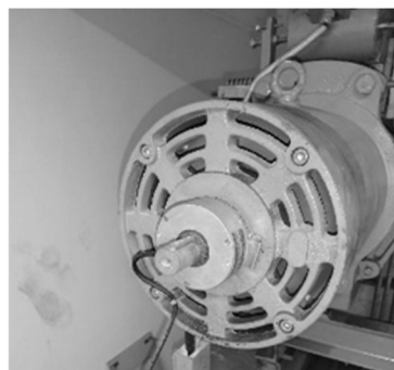
Figure 7. No electrical switch
