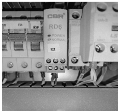
Figure 9. Electric relay damage
